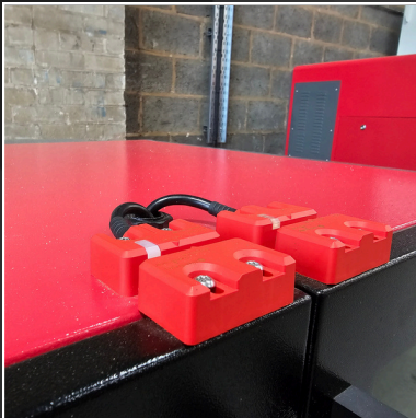
Allen Bradley Safety Interlocks
