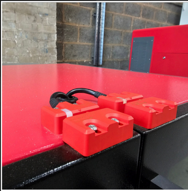
Allen Bradley Safety Interlocks
